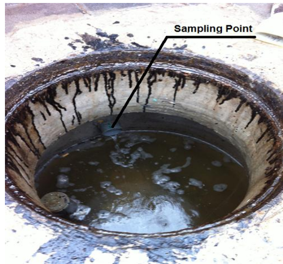
Figure 3- 5 Sampling Point of Rooftop Runoff
